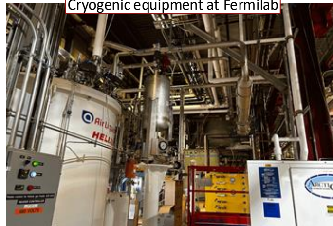
Cryogenic equipment at Fermilab
