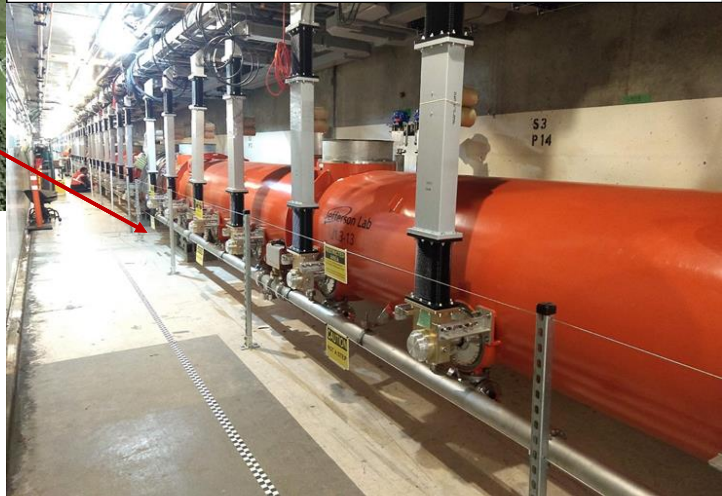
View of superconducting cryomodules in the LCLS-II tunnel
