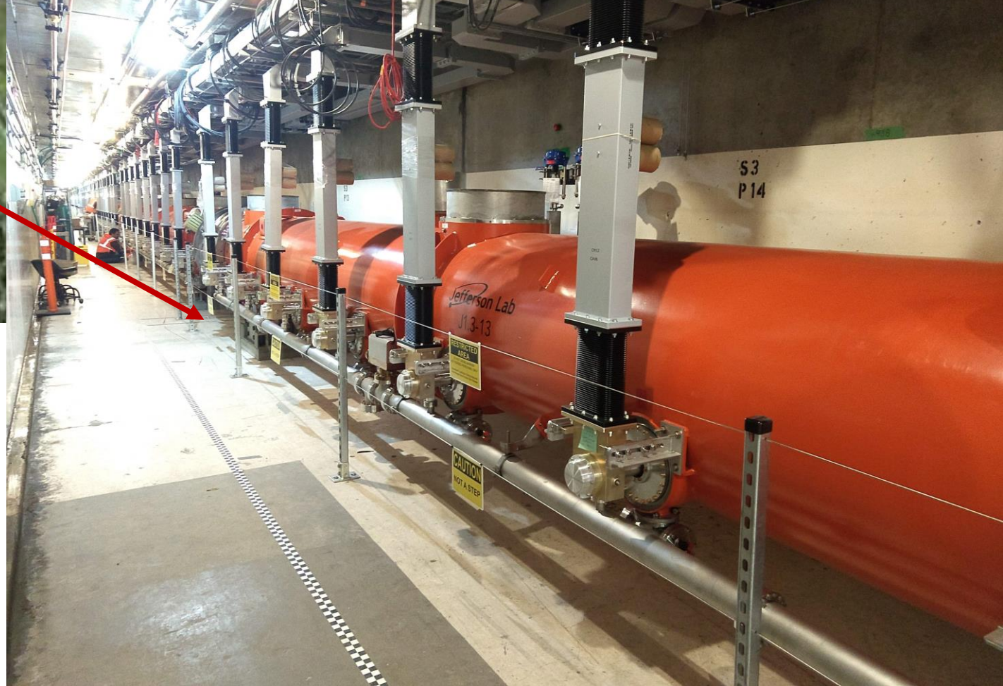
View of superconducting cryomodules in the LCLS-II tunnel
