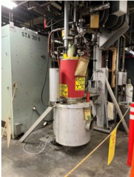
Klystrons Produces prompt X-Rays from gaps in shielding
